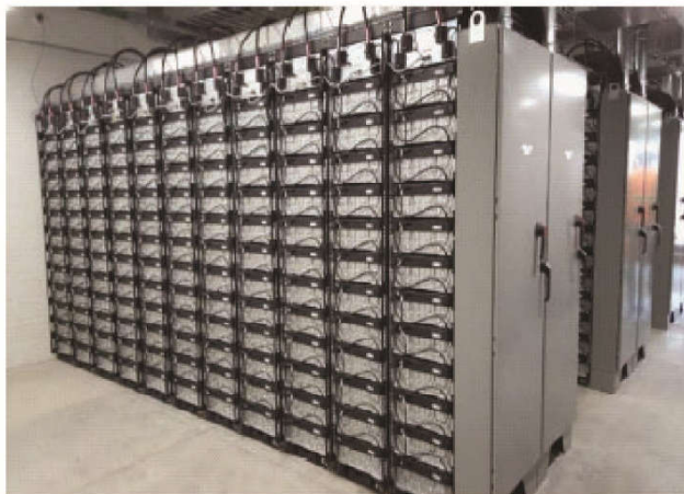
Battery Energy Storage
